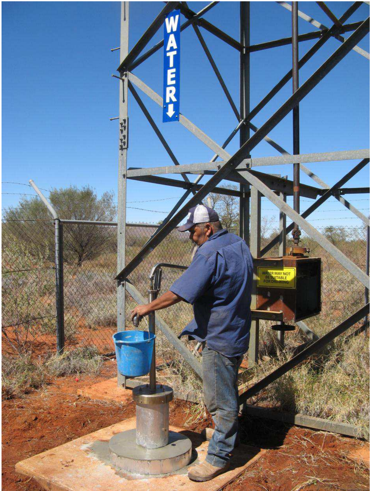
Mt Barkly hand pump installed by Centre for Appropriate Technology
